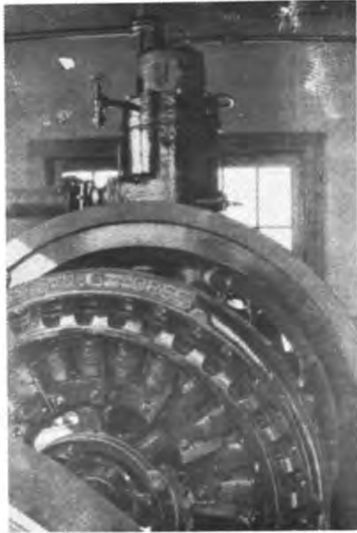
NBD - Radioman Ted Hancock's "Pride & Joy" -- The Standby power plant at Seawall !
